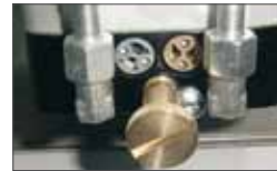
By pass valves Valvole by pass
